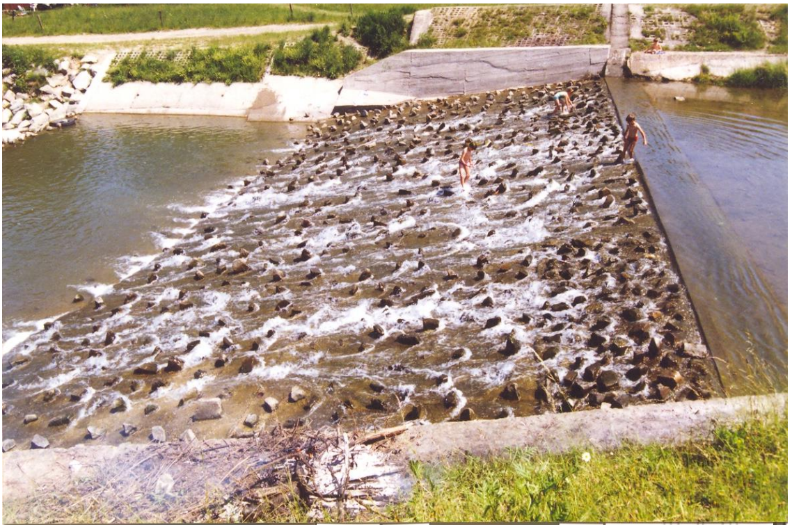
Photo 4. Photo of the rapid hydraulics structure after the rebuilding (photo by A.Radecki-Pawlik).
