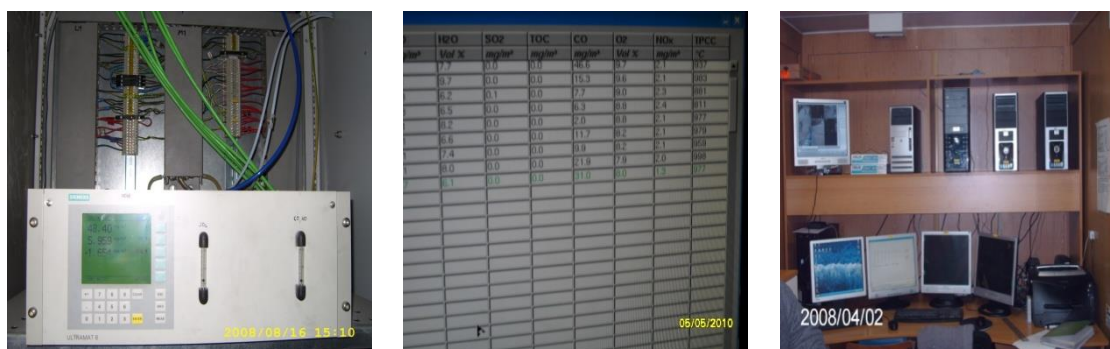
Figure 5 S.C.A.D.A. Automatic System (Control System and Data Collection) (Photo: Ana Humeniuc).
