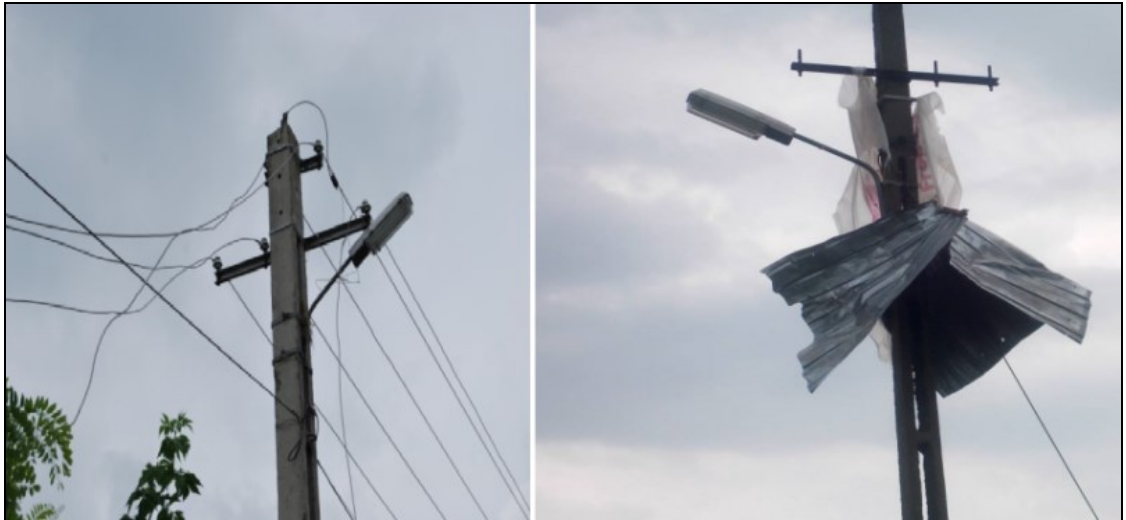
Figure 6 Broken steel bar (left), and a roof carried by the wind over a distance of circa 150 m (right).
