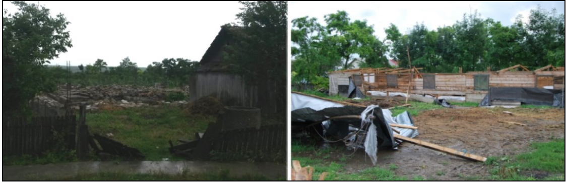
Figure 4 Concrete outbuilding with destroyed walls (left), and outbuilding with roof lifted by wind and carried 50 m (right).
